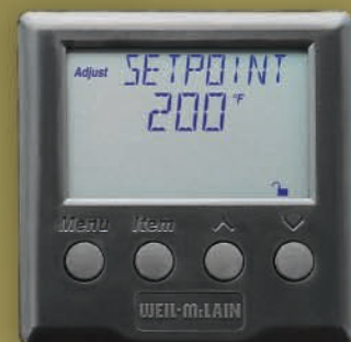
Set Point Operation
